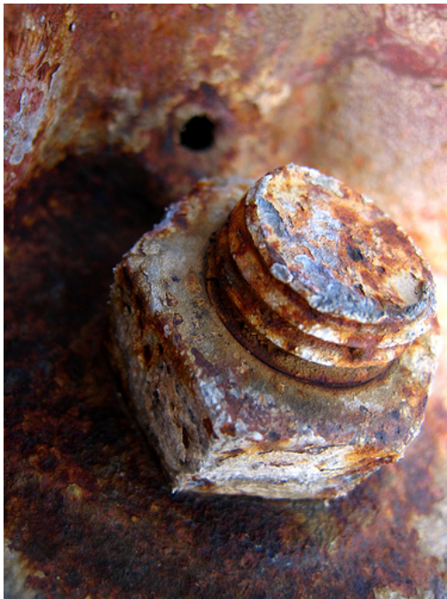
Florida, USA - failure of coating after 6 months
